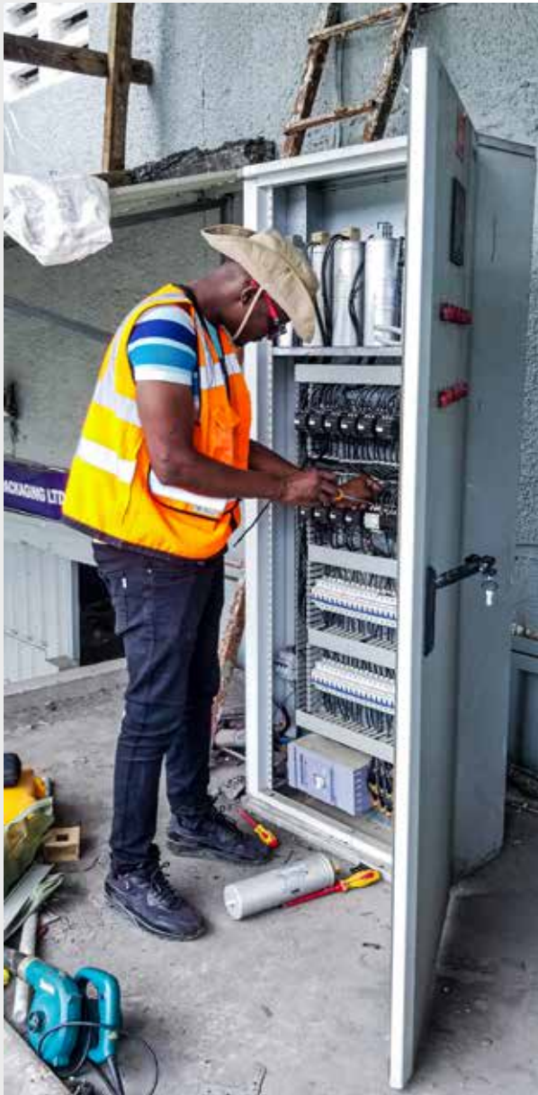
Power Factor Correction Service at Creative Packaging Ltd Chang'ombe , Mbozi Rd Dar es salaam
