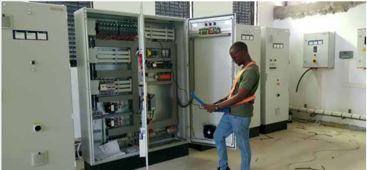
340kw Power distribution House Panels installation and PLC programming at Hill group Ltd Bagamoyo Pwani Tanzania
